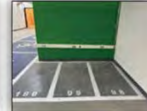
Electric Scooter Charging Area
