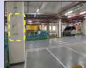
EV Charging Spaces with Power Reserved
